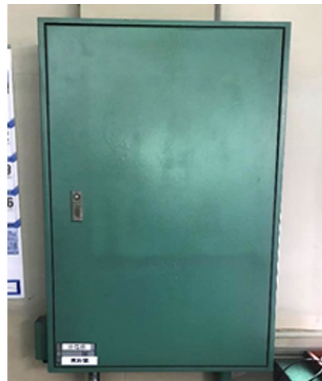
Automatic control panel
