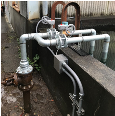
Water discharge control valve
