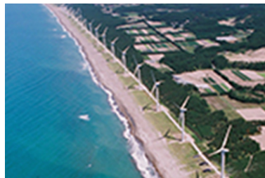
Hachiryu Wind Farm
